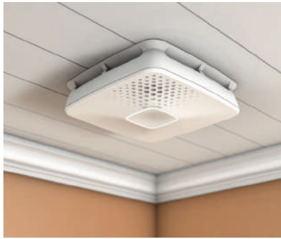
(a) Smoke detector
